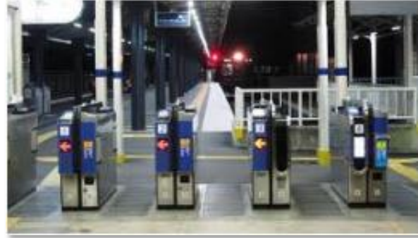
Automatic gate system
